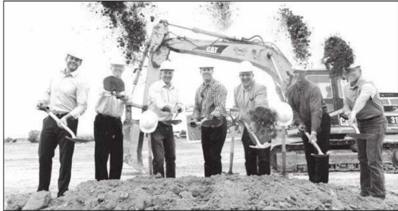
Brinkman Partners and city of Fort Collins representatives, from left, Josh Guernsey, Darin Attebury, Brian Stahl, Kevin Brinkman, Wade Troxell, Jay Hardy and Todd Parker throw dirt at the Harmony Commons groundbreaking June 30 in Fort Collins. Harmony Commons is an upcoming mixed-use development that will include retail, office and hotel uses.
